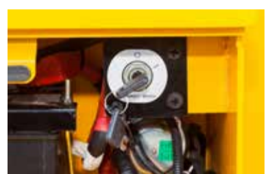
Battery master switch
