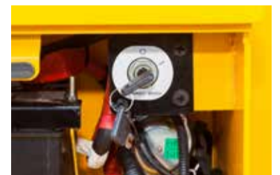
Battery master switch
